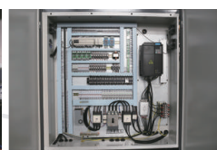
HT & HTS-电气系统 HT & HTS-Electrical System
